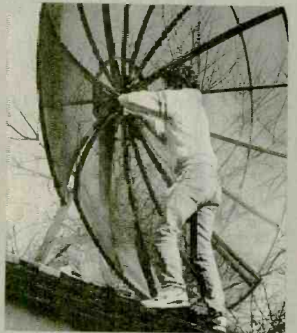
The fourth section is mounted in place. We found it easier to hang it in place before fastening it to its neighboring petals.
