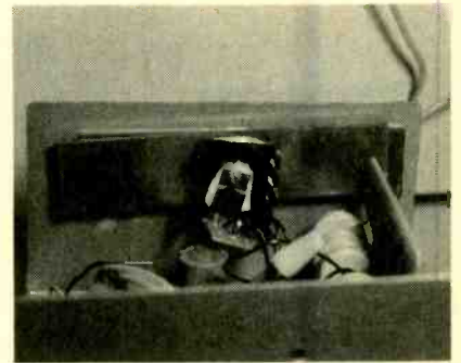
Select a metal (TO-220) package for Q2, and mount it to the side of the enclosure as shown here.
