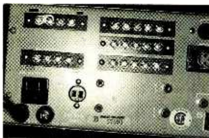
Professional systems have provisions for 25-volt and 70-volt constant-voltage speaker lines. The set of screw terminals in the upper left corner of this amplifier are the constant-voltage outputs.
