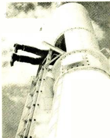
Difficult position is required of technician shown here working on the bearings of a TACAN rotating antenna assembly.
