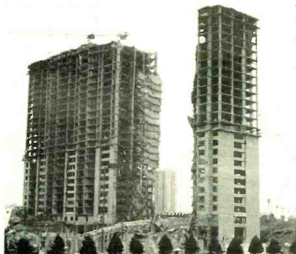
This is the site of the high-rise disaster, where a crane fell and brought down a whole section in the middle of the building under construction. Scene is Bailey's Crossroads in Virginia. Rescue operation was speeded by Fairco REACT.
