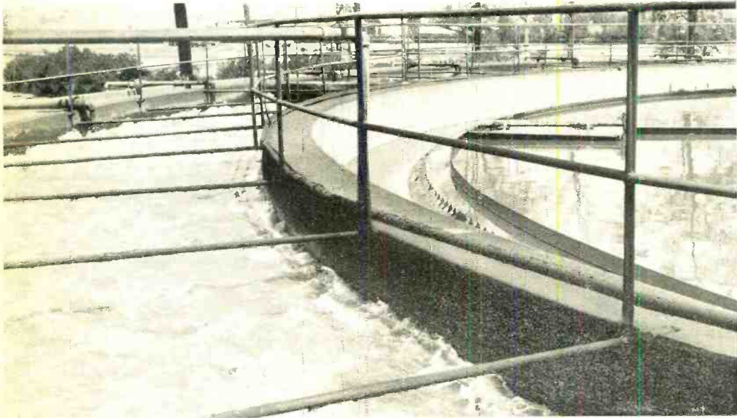
Fig. 1. Skimming and aeration system at a water treatment plant.
