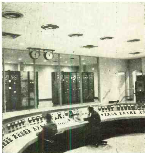
The Master Control Panel at the receiving station of the USIA's new broadcast complex at Greenville.
