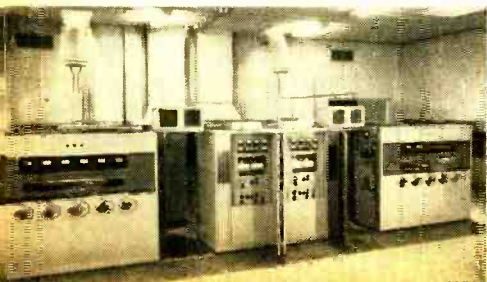
New 100-kw. transmitters for Radio Australia. Located at Shepparton, units handle programs for stations VLB and VLE.
