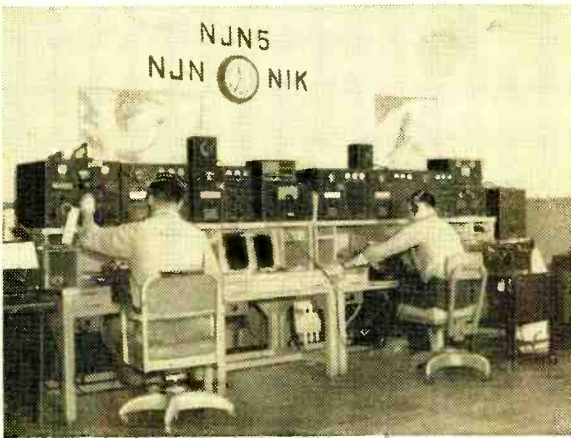
A typical USCG shore station radio installation is the International Ice Patrol HQ at Argentia, Newfoundland.
