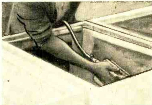
Acoustical lining , requisite in bass reflex enclosures, is fastened by air-pressure stapling gun.
