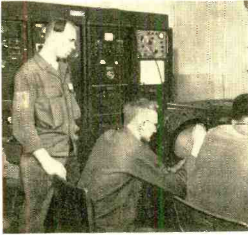
Electronic equipment shown above is installed in one of the gap-filler radar stations which are located between more powerful long-range search transmitters.
