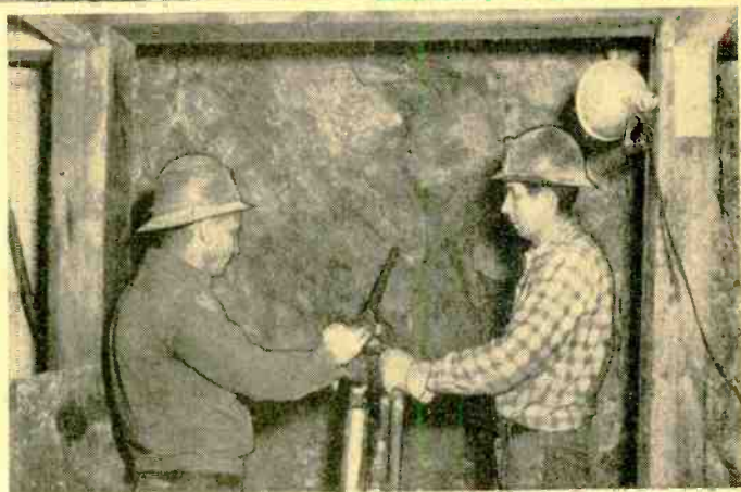
Joe Mosbrucker, on the left and Tom Gribbin set up a jack-leg drill in the Miracle Mine. At this writing, it was the only California mine to have shipped out a carload of commercial uranium ore.
