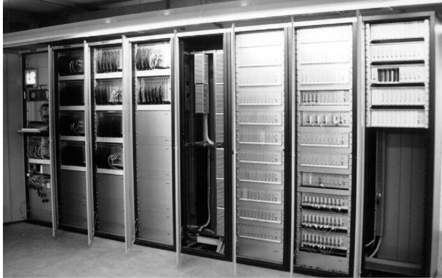
The large Plettac CCTV matrix at Frankfurt Airport
