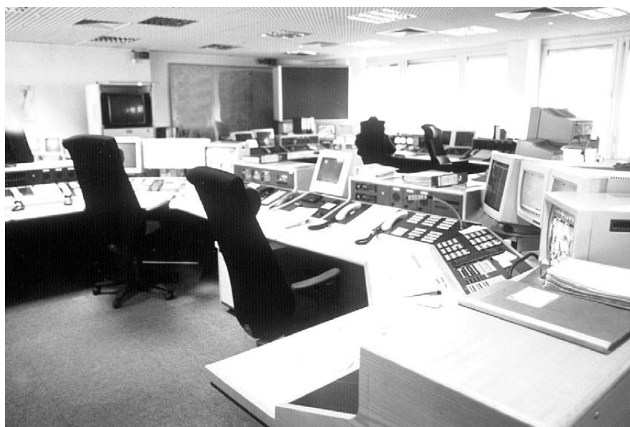
A well-designed control console
