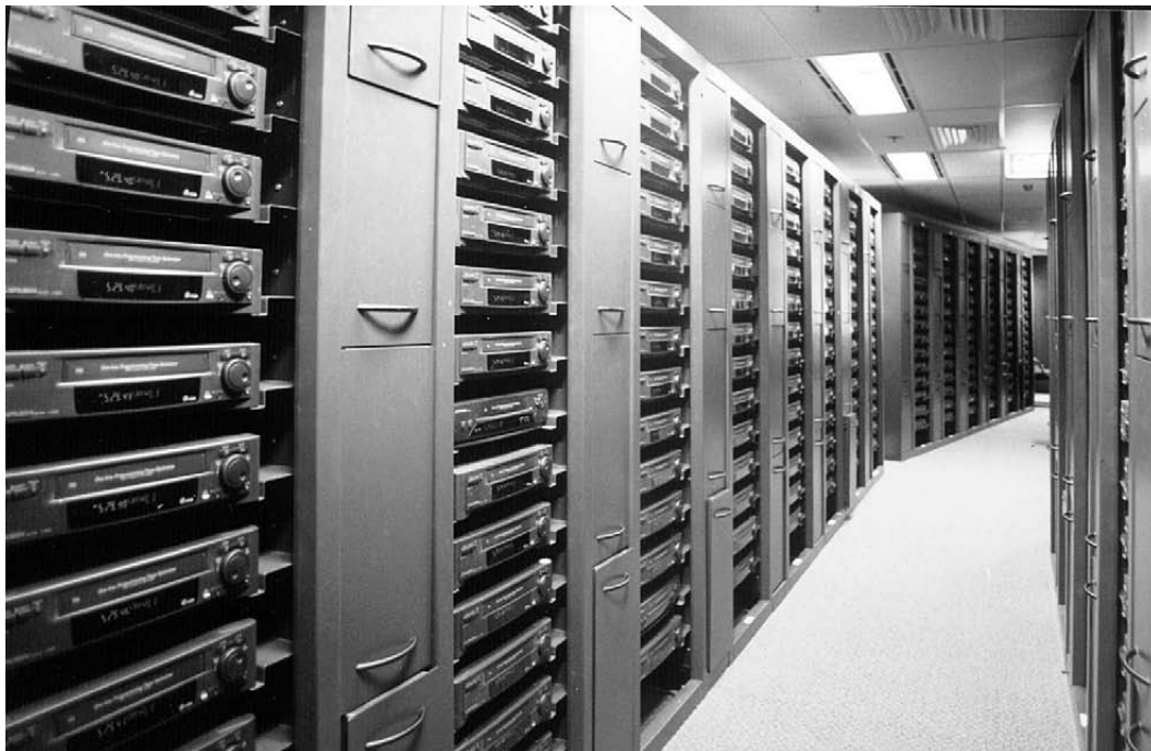
Walls of VCRs in Sydney's Star City Casino record all cameras in real time mode, fully managed by the matrix switcher.
