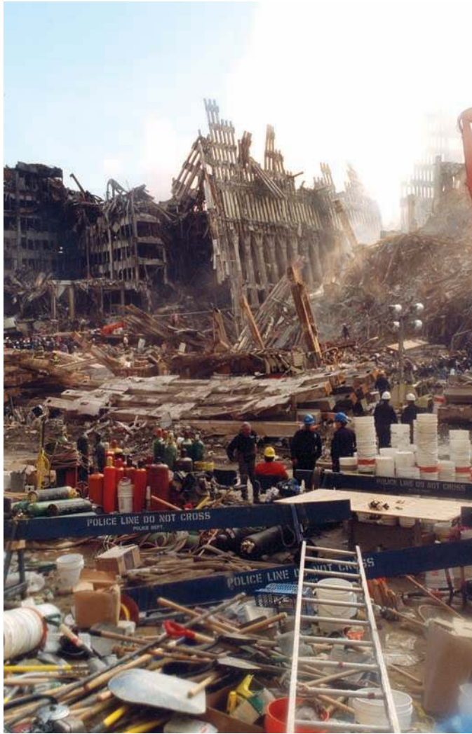
Figure 10.7 GROUND ZERO WORLD TRADE CENTER. This photo illustrates the extensive destruction from the collapse of the two World Trade Center towers. It also depicts the massive search and recovery operation. (Courtesy of retired Detective First Grade Kurtis Harris, NYPD Crime Scene Unit.)
