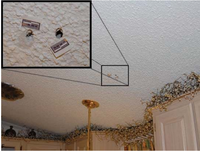
Figure 3.10 Above the sink are two defects in the ceiling. The defects are consistent with bullet holes. (Photo courtesy of Chuck Merritt, San Diego County Sheriff's Office.)
