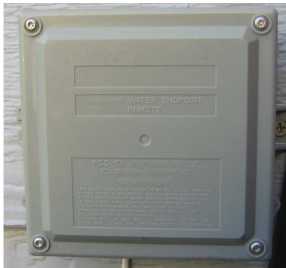
FIGURE 7.2 A remote monitoring sensor for utility usage.
