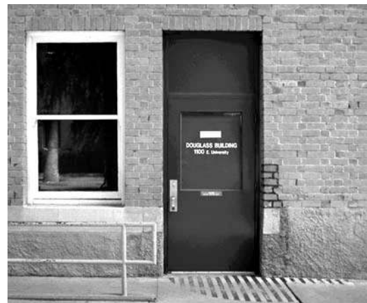
Figure 19.7 Door swinging into a walkway.
