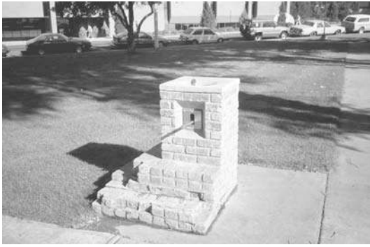
Figure 19.8 Abrasion on masonry steps.
