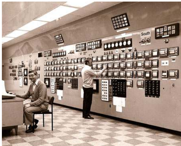
Fig. 8.1 A typical conventional panel from a process plant operating in the 80s
