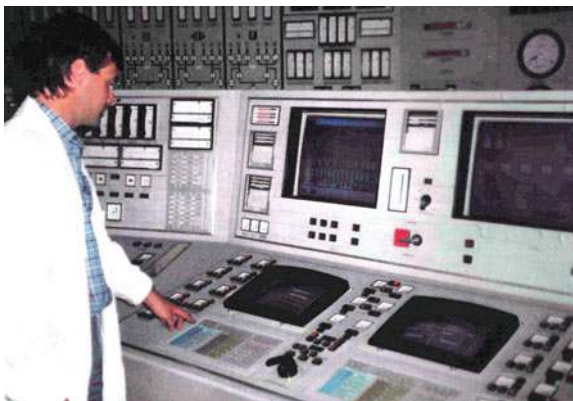
Fig. 8.4 The NORS simulator console showing 1980s advanced controls
