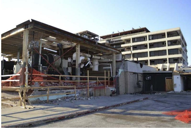
FIGURE 9-8 Joplin, MO, August 3, 2011 — Damage sustained at St. John's Regional Medical Center after the May 22 EF-5 tornado that struck the city. FEMA is working to provide assistance to those affected by the tornado. (Source: Photo by Elissa Jun/FEMA)
