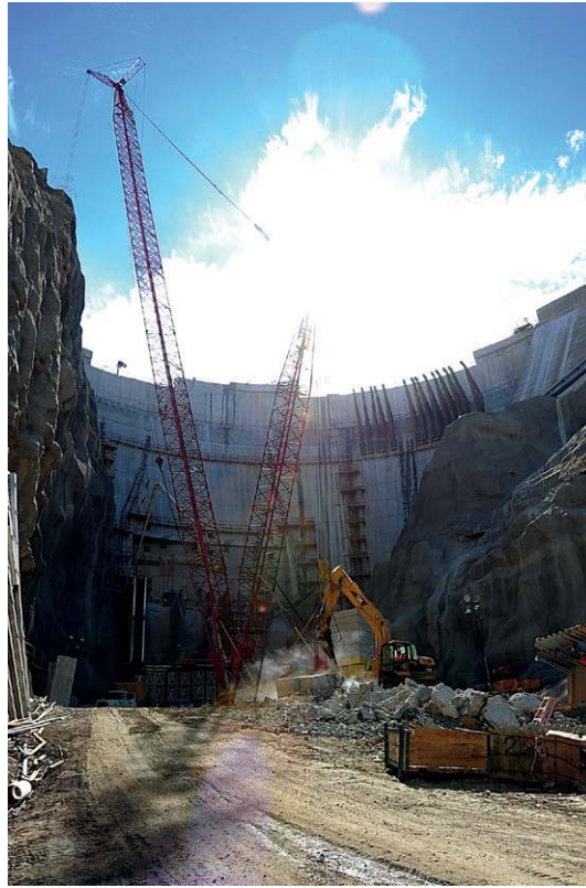
FIGURE 8–2 La Canada Flintridge, CA, August 2, 2010 – The Big Tujunga Dam is under construction to reinforce the walls due to an increased debris flow from recent severe winter storms. Under the declaration DR 1884 for Public Assistance, FEMA funds emergency protective measures for critical infrastructure such as roads, bridges, and dams. (Source: Photo by Adam DuBrowa/FEMA)
