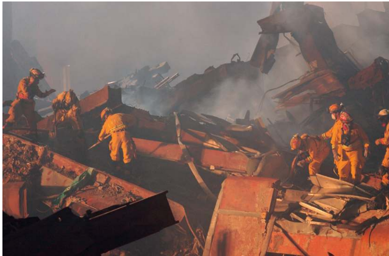
FIGURE 9–11 New York City, NY, September 21, 2001 — Rescue operations continue far into the night at the World Trade Center. (Source: Photo by Andrea Booher/FEMA News Photo)
