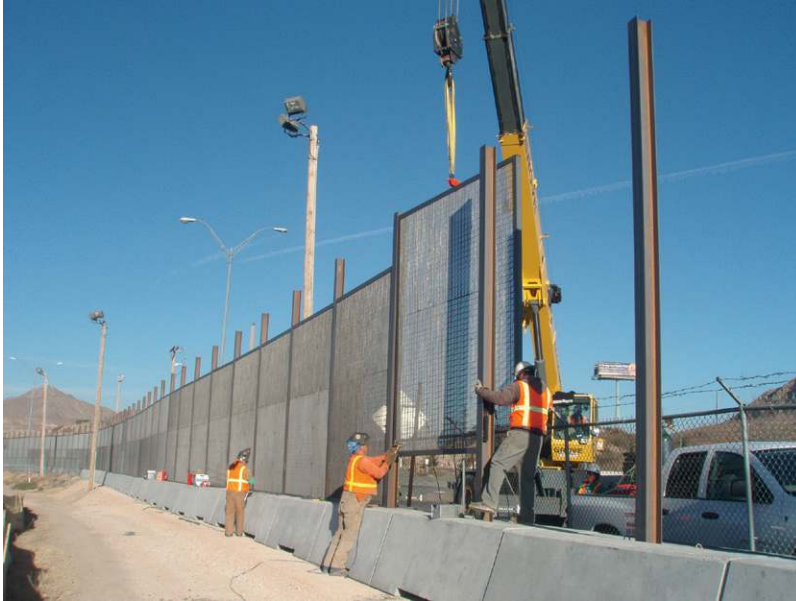
FIGURE 6-3 Cerrudo services construction workers assemble the southwest border fence in El Paso. (Source: CBP, 2011)
