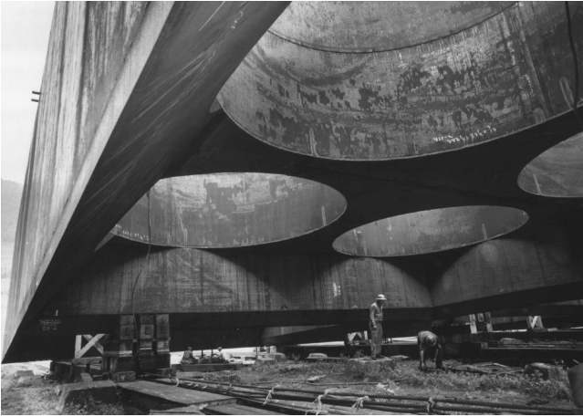
Underside of open caisson for Greater New Orleans bridge over Mississippi River. (Dravo Corp.)
