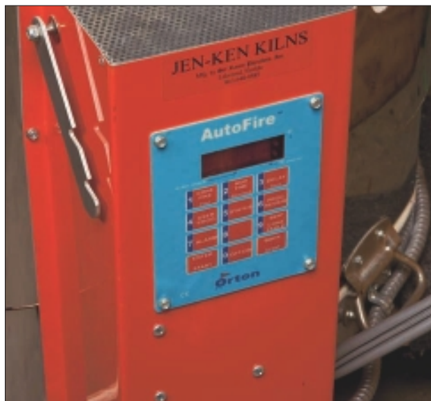
Figure 13-2: Automatic controller mounted on a glass kiln.
