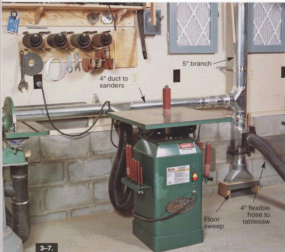
Sharing duties reduces duct length. Here, one 5" branch serves the tablesaw, floor sweep, and a 4" pipe to two sanders. Blast gates direct airflow to just the ports in use.
