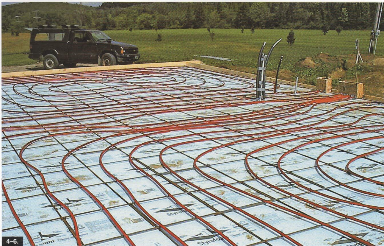
In a radiant-slab floor, heated water flows through flexible plastic tubing that gets routed and secured before pouring concrete. Electric in-floor radiant systems exist, as well.
