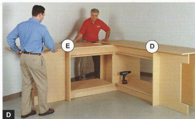
Position the long and short tops (D, E). Drill pilot holes, and screw them in place.
