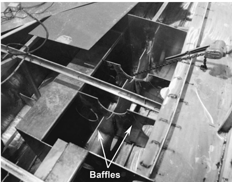
Figure 5-13. Baffles in aluminum tank
