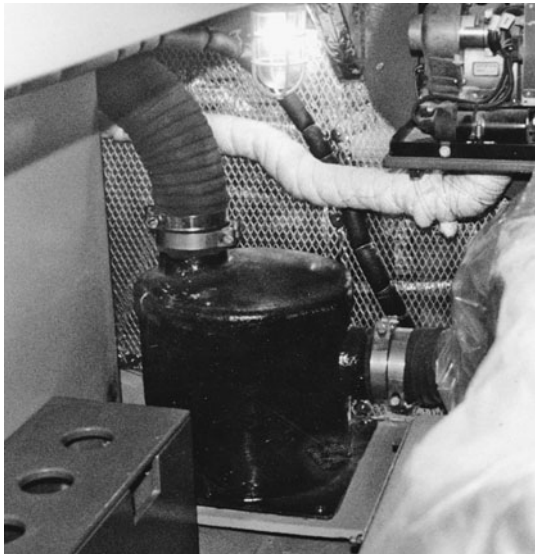
Figure 7-11. Waterlift muffler installed
