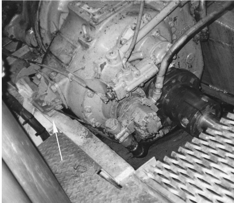
Figure 3-5. Engine installed on rigid mounts
