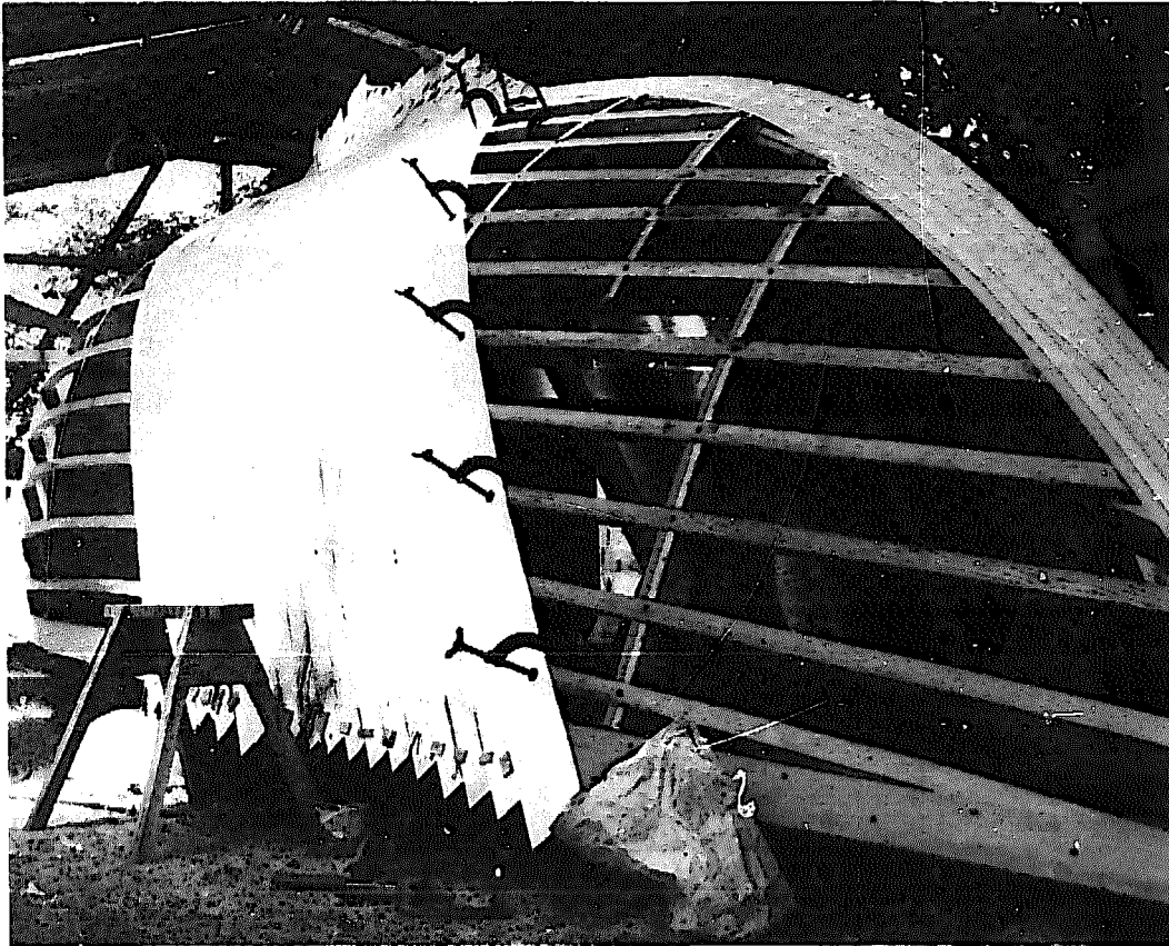
Figure 11-15. The first skin being applied to a framework of molds, bulkheads, and stringers. (Photo courtesy of John Guzzwell.)
