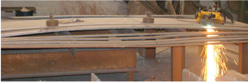
Fig. 11.5 Edge buckling due to oxy-acetylene cutting
