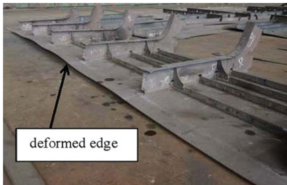
Fig. 8.3 Deformed edge leads to misalignment during panel assembly
