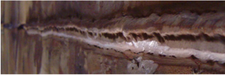
Fig. 19.5 A severe case of longitudinal crack
