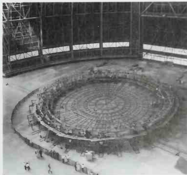
On the floor of the hangar, workers finish assembling one of the Akron 's main frames. When it was completed, the 36-section ring was hoisted into a cradle for joining to the longitudinal girders.
