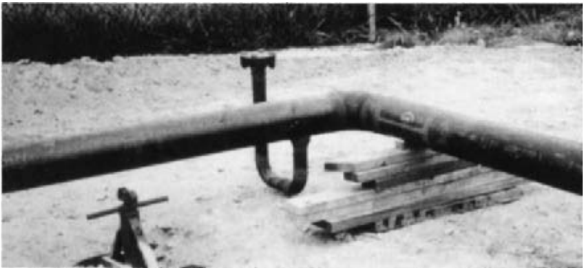
FIGURE B13.97 Example of a low-point leak-detection sump in a metallic fuel oil system.
