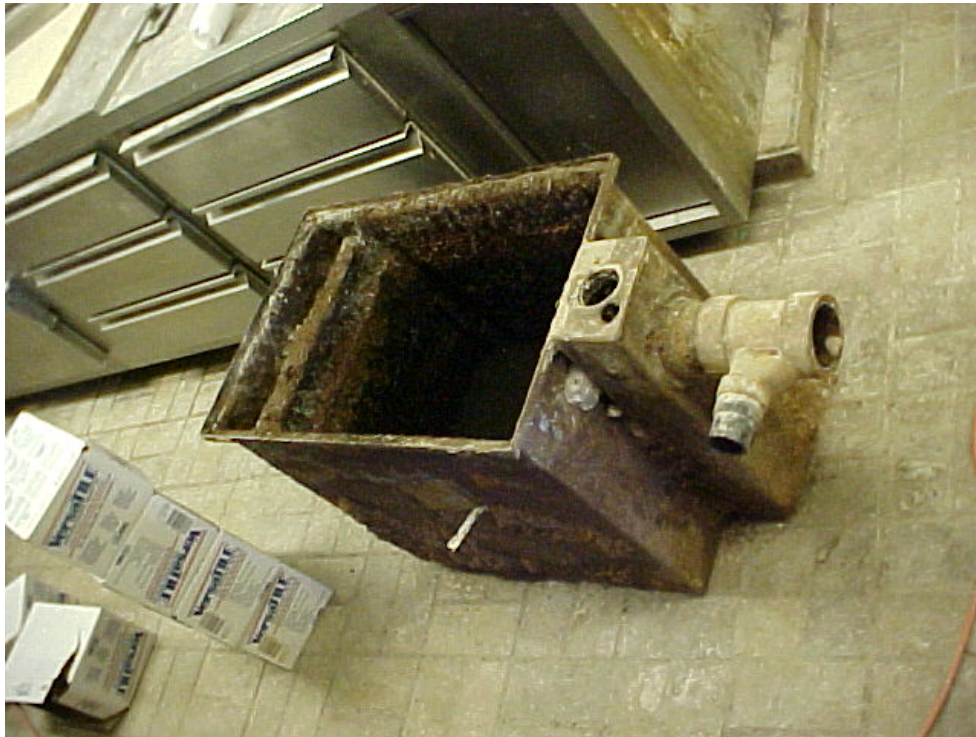
Common and worn out kitchen Grease Trap. The grease contains lots of acid and this acid will eat metal as with this grease trap.
