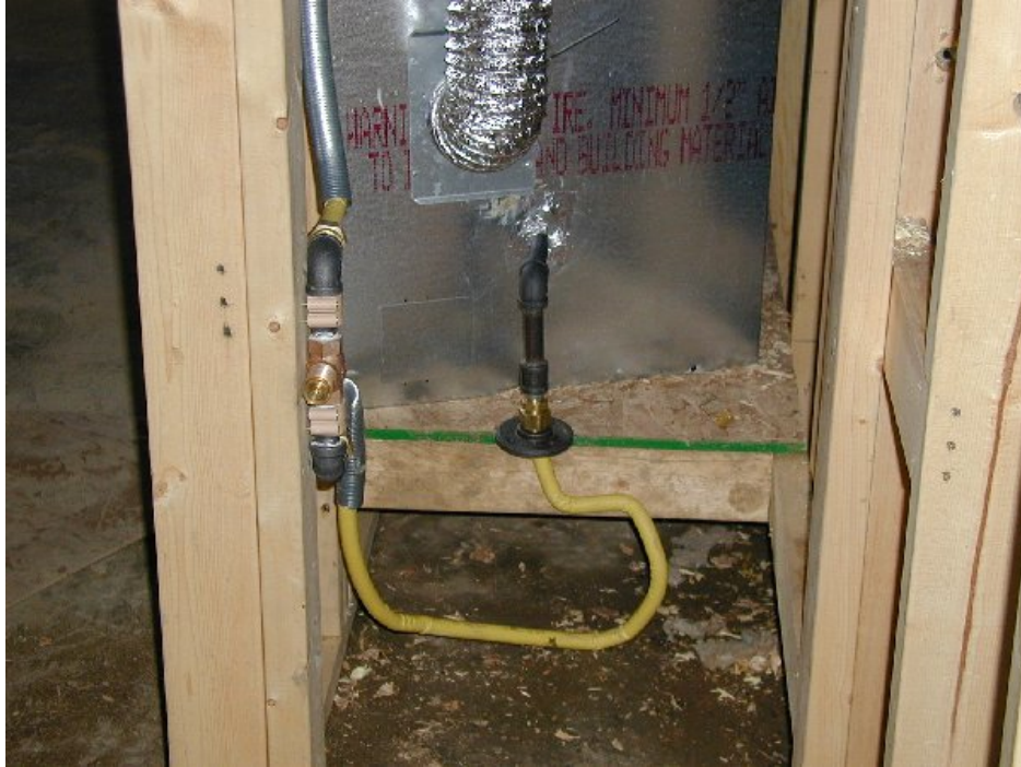
Gas manifold and connector to a fireplace.
