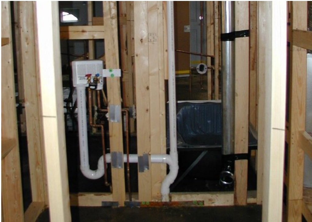
Suds producing fixture 2 inch VTR Vent through Roof and Trap.
