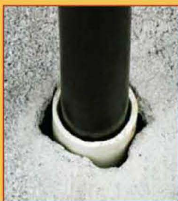
59 | Sleeving the Pipe
