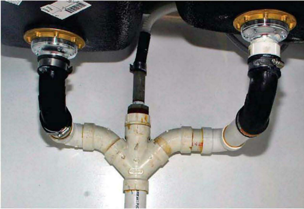
My custom drain system installed under a sink. The lower pipe feeds into the trap.
