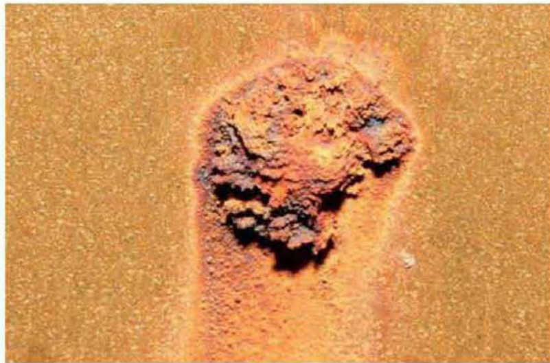
Seen inside the heater is a rusted-through leak spot. This corrosion, the size of a penny, ate through the steel jacket to spring a leak.
