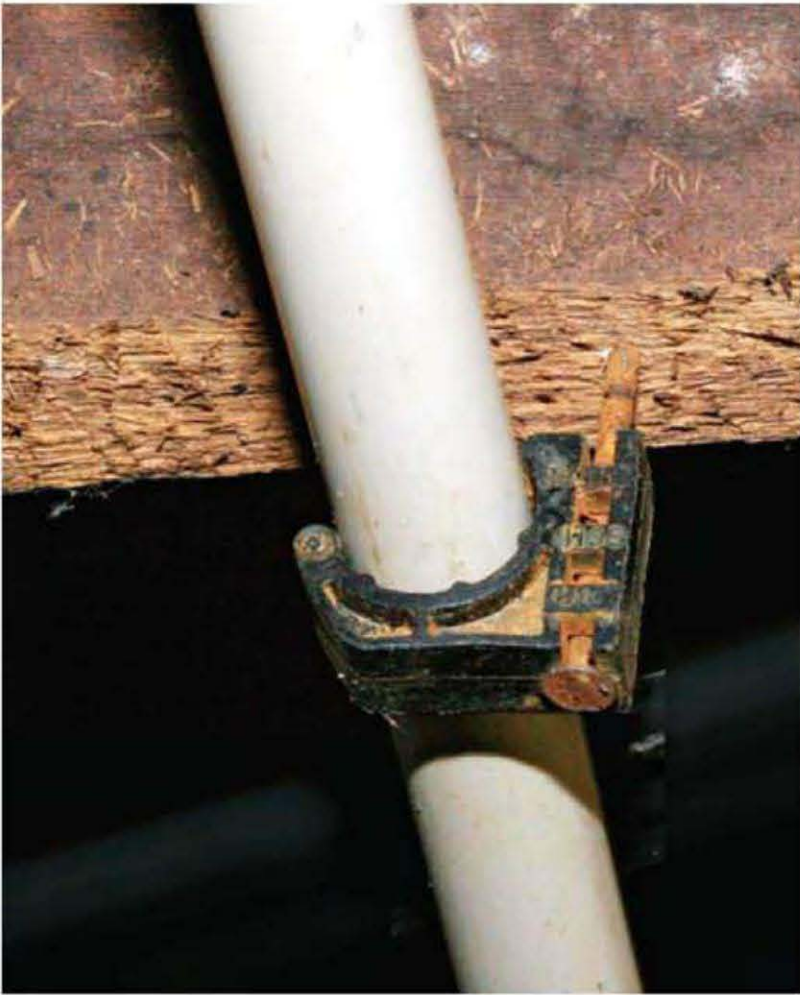
Tube talons like this one are a good option to secure a single pipe though they are relatively expensive.
