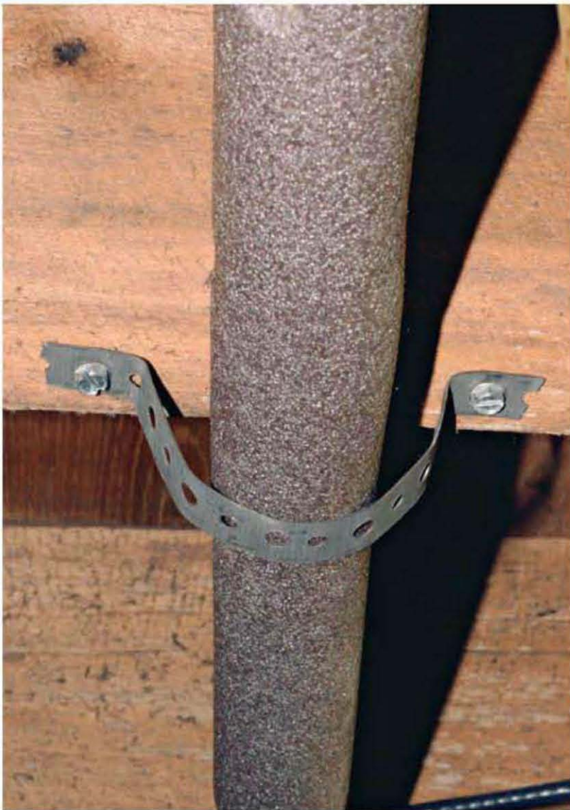
My favorite method of securing insulated pipe is with common metal strapping. It is fast and inexpensive.
