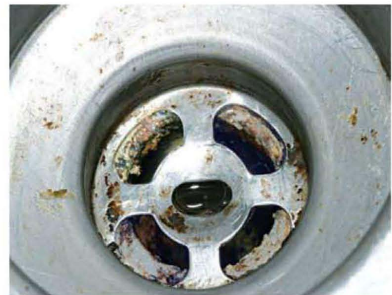
Gaskets like this (top), with a flat top extending into the drain right under the strainer, are commonly used. These sometimes cut the drain flow by 50 percent. They also catch food particles and provide a breeding ground for bacteria (bottom).
