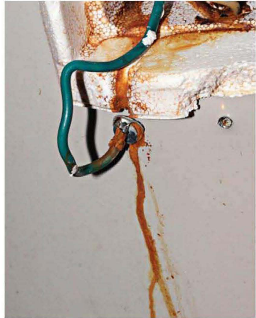
The orange streak is an indicator of another water heater heading to the land fill due to a tank leak.
