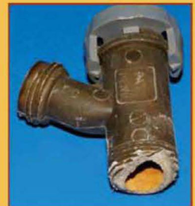
126 | Unclogging Drain Valves
