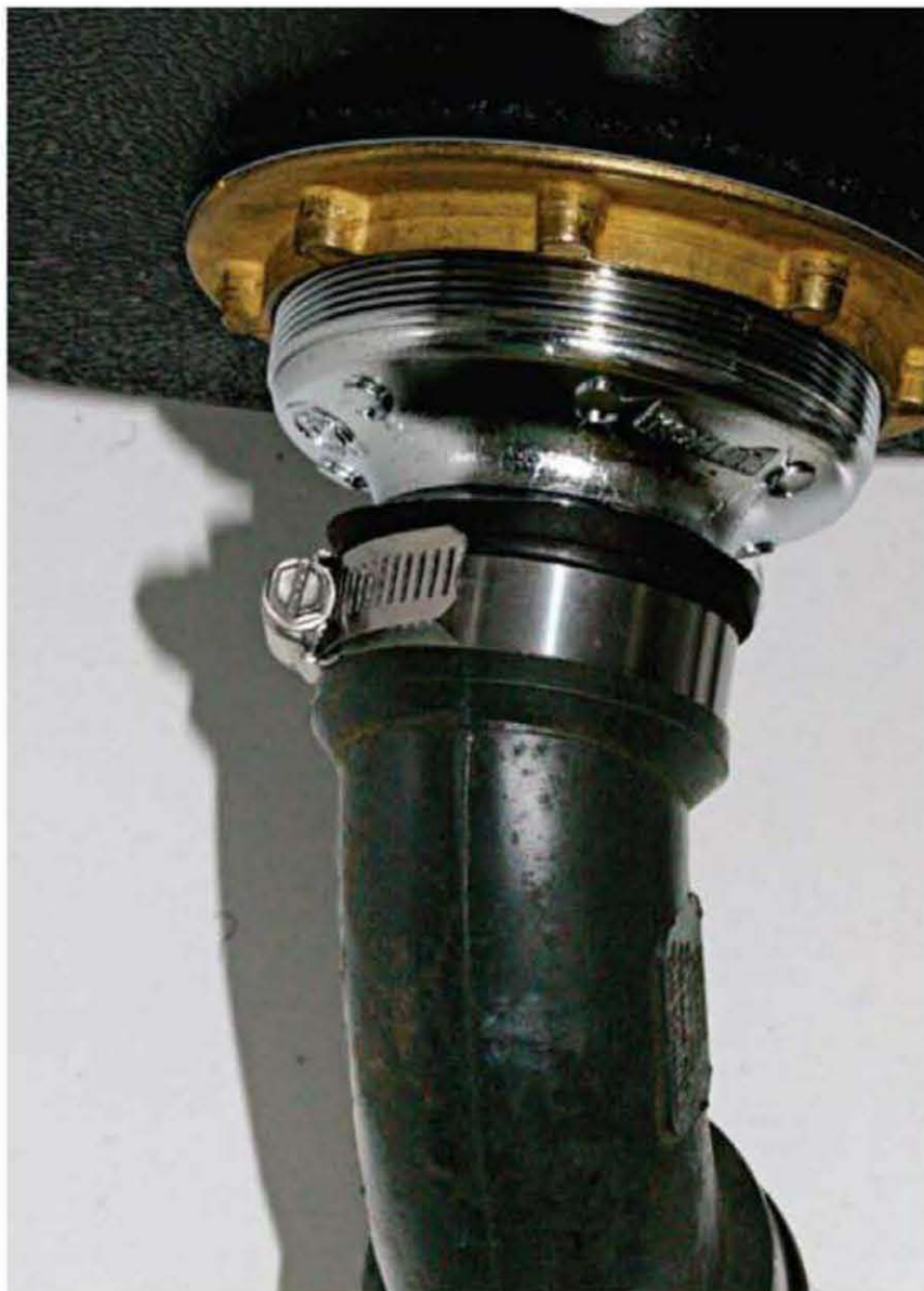
I connect the strainer to the drain assembly with a Fernco flexible elbow and point it toward the back wall. Grabbing onto the outside of the threads, and eliminating the gasket that extends into the pipe allows a full-flow output within the strainer drain.
