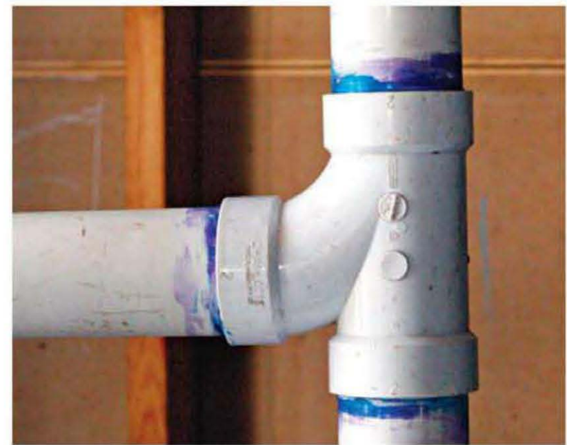
Vent-only Ts should be installed upside down to allow better airflow from horizontal to vertical.
