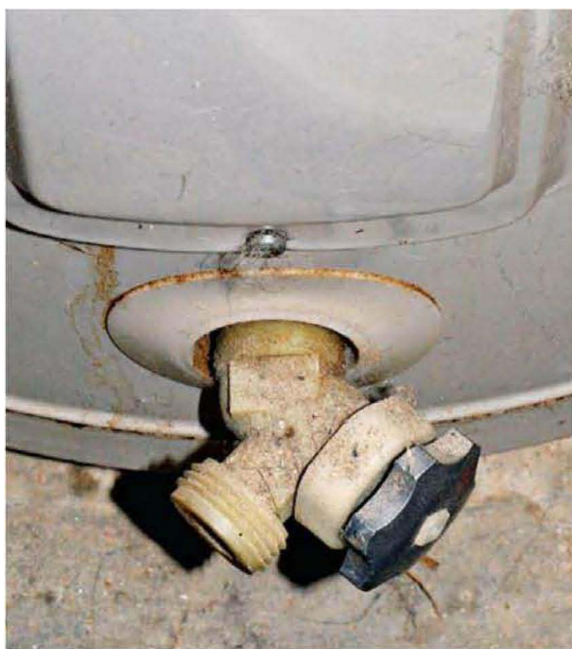
Opt for brass drain valves and avoid plastic ones like this. Brass is always superior to plastic.
