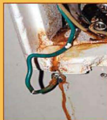
127 | Finding Water Heater Leaks
