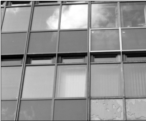
Figure 6.6 Several refurbished panels (left) demonstrate the improvement compared to the adjacent existing panels (right)
