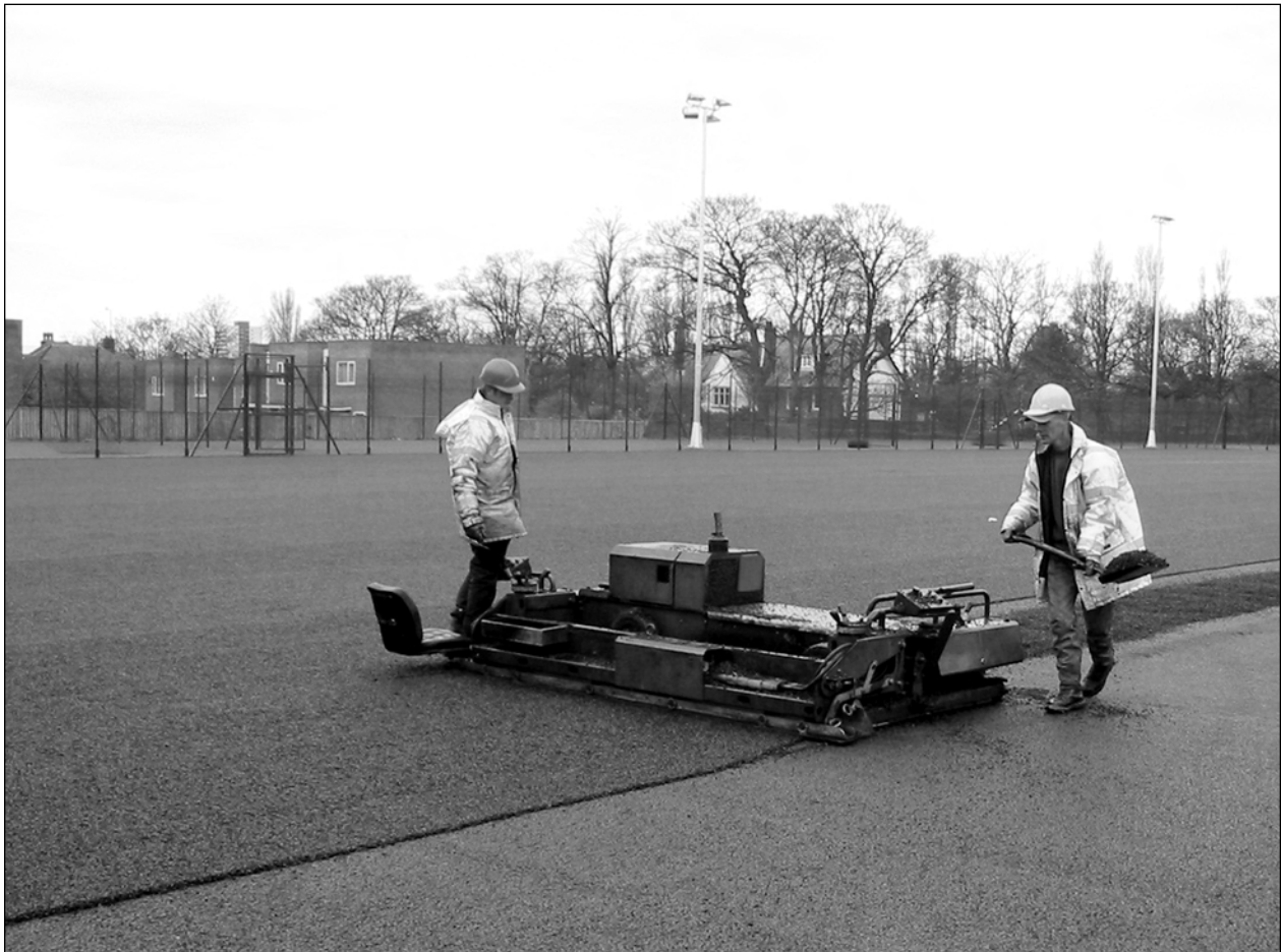
Figure 7.4 Rubber recycled from car tyres being laid to form an artificial surface for outdoor sports
