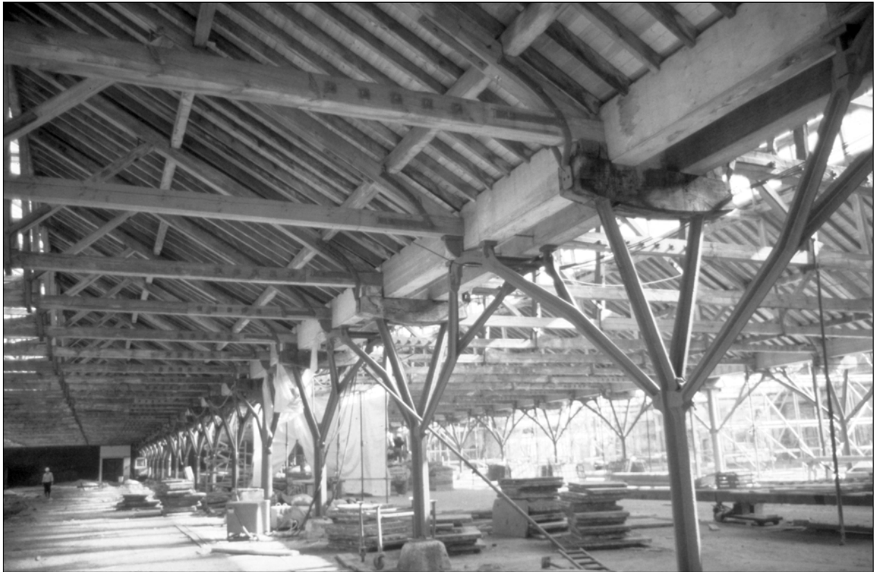
Figure 4.4 Tobacco Dock, East London, UK (1812–13): The 17-metre-span (54 feet) timber roof trusses are supported on cast-iron columns resting on granite vaults resting on timber piles
