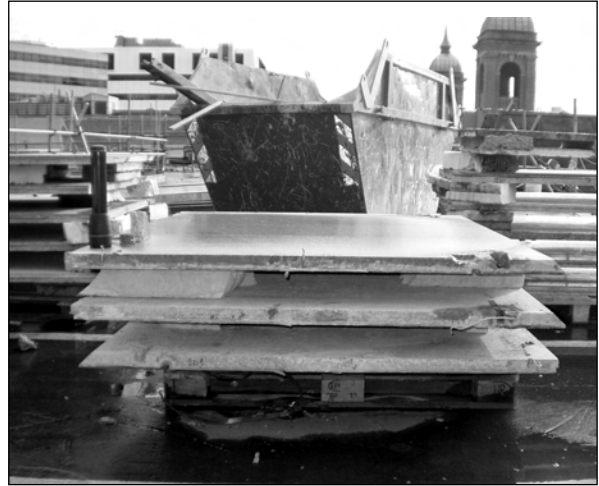
Figure 6.7 Queen Street Place, London, UK: Granite panels removed from the original façade
