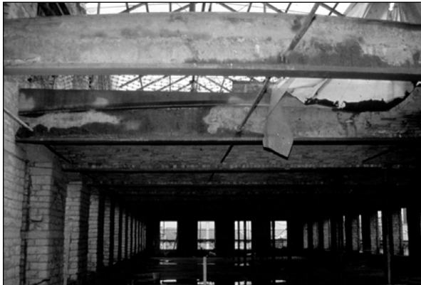
Figure 2.16 Jack arches were removed in some bays to provide space for new staircases and services risers
