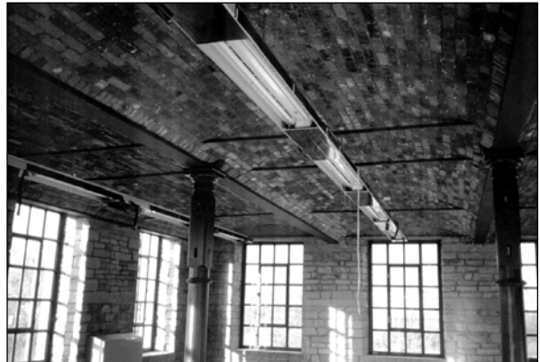
Figure 2.17 Interior of the refurbished building showing new windows, cleaned jack arches and exposed structure
