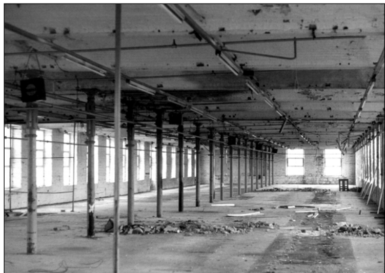
Figure 2.14 Interior of the disused mill prior to reuse of structure and refurbishment
