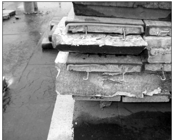
Figure 6.8 The stainless-steel fixings were also inspected and reconditioned or replaced, as necessary
