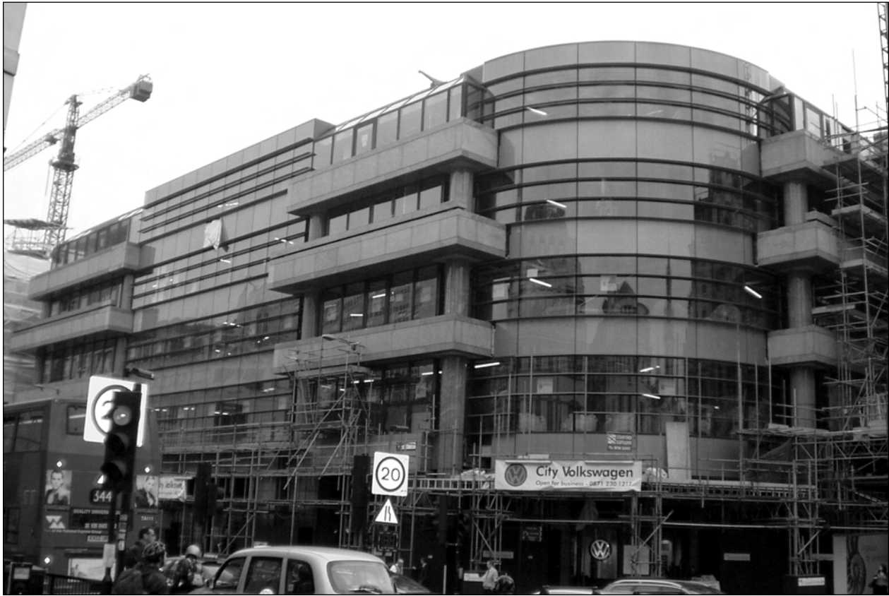
Figure 6.9 The new granite façade nearing completion, flanked by the reglazed aluminium framed windows
