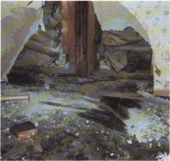
Figure 7 Detached mineral fibre insulating blankets
