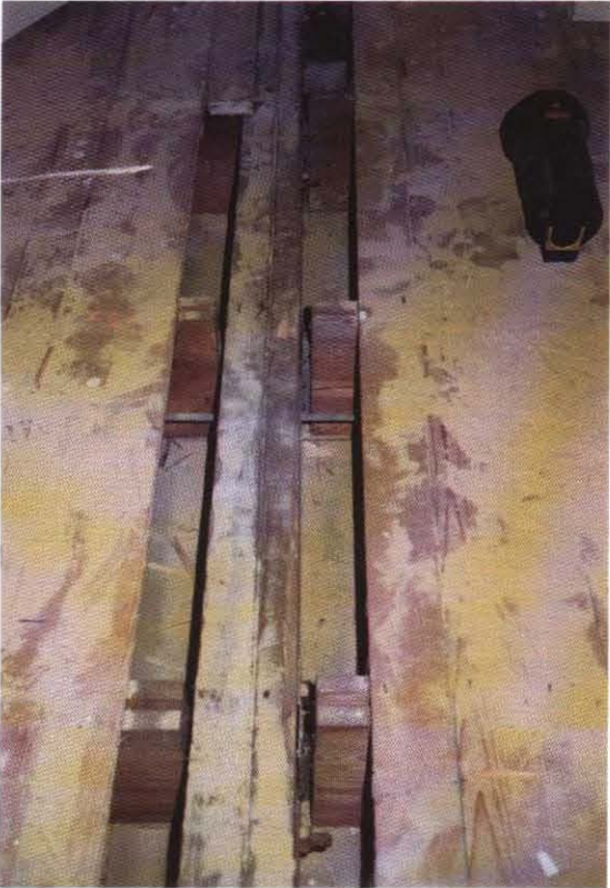
Figure 8 Wide gaps between the ends of joists and joist hangers
