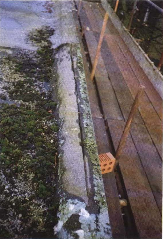
Figure 9 Crack between the asphalt roof cover and aluminium flashing
