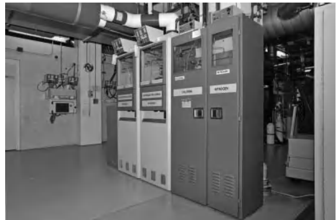
FIGURE 23-6. View of Ventilated Toxic Gas Cabinets.
