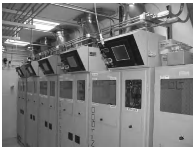
FIGURE 23-9. View of ventilated toxic gas cabinets.
