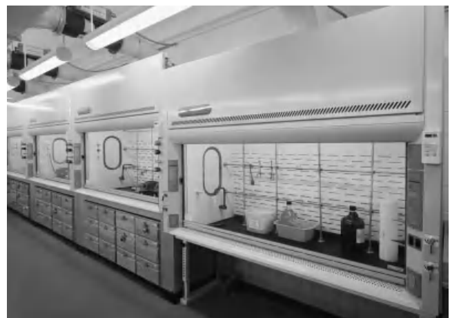
FIGURE 2-6. ADA accessible fume hood in a teaching laboratory. (Courtesy: LabConco, Corp.)
