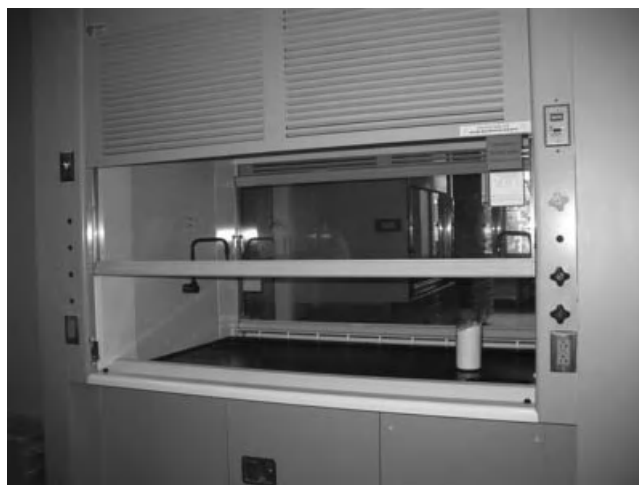
FIGURE 16-6. View of a pass-thru chemical fume hood.
