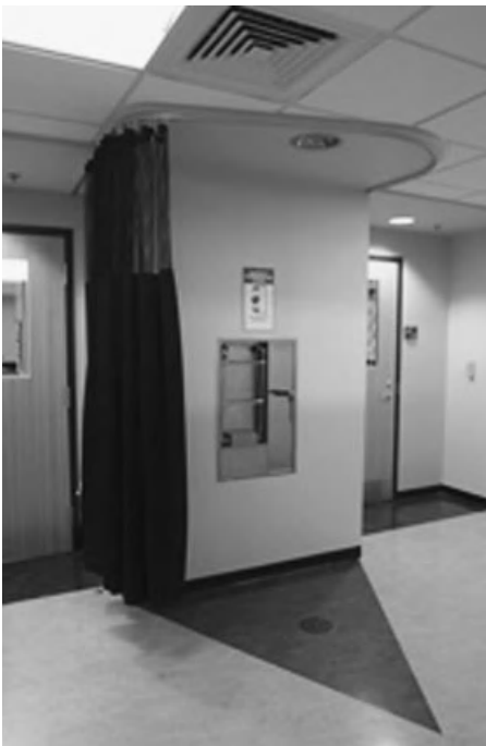
FIGURE 2-11B. View of emergency eyewash and deluge shower in a corridor (Copyright by HERA Laboratory Planners).
