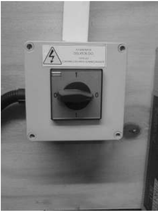
Figure 10-42 Mains isolator switch.
