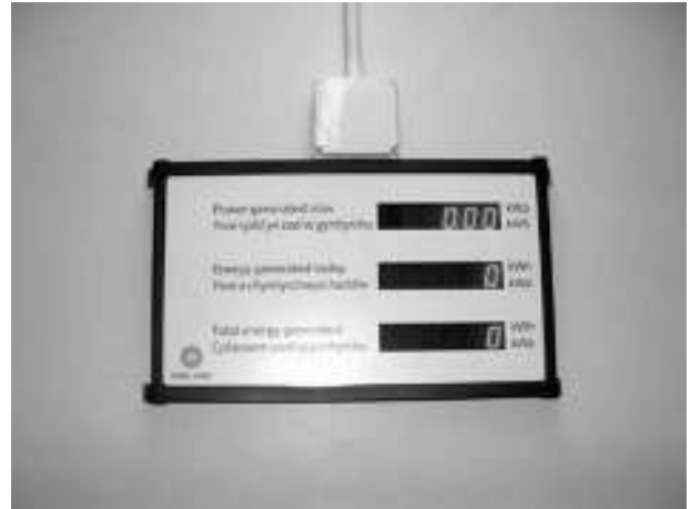
Figure 10-46 Awelamentawe school solar display. Image courtesy Dulas.
