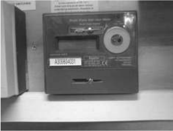
Figure 10-45 Watt hour meter.
