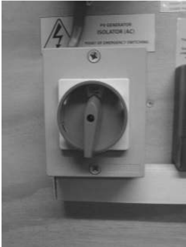
Figure 10-44 Solar DC isolator switch.
