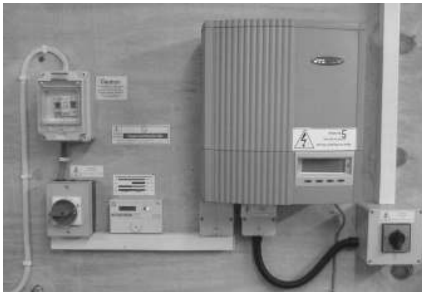
Figure 10-41 A typical inverter setup.
