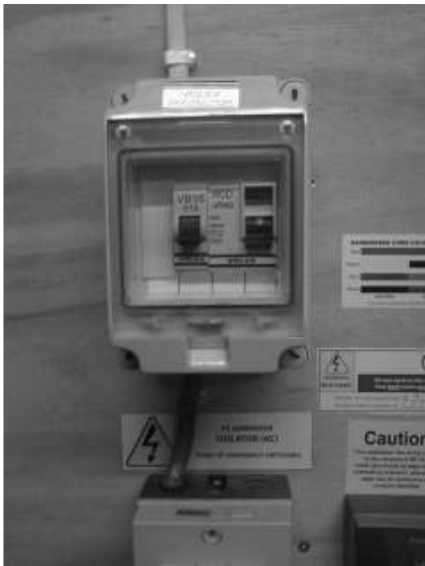
Figure 10-43 Mains circuit breaker.
