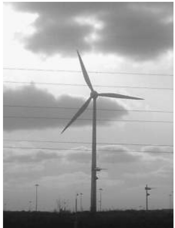
Figure 2-7 A wind turbine illustrating the power we can harness from the wind.
