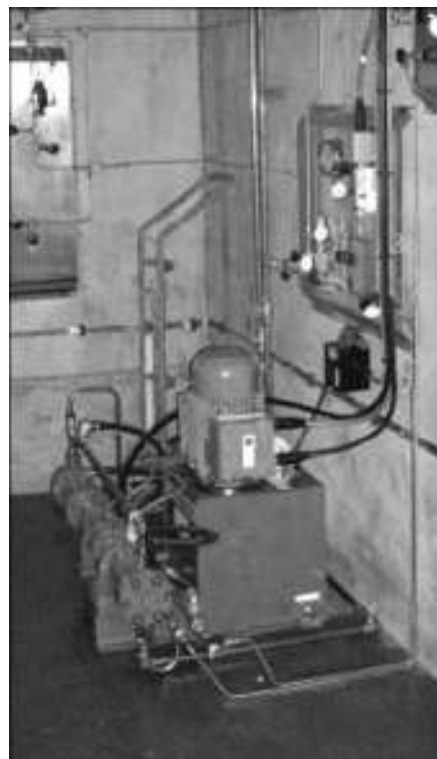
Figure 4-25 Hydrogen compressor at HARI project, West Beacon Farm. Image courtesy Dr Rupert Gammon.
