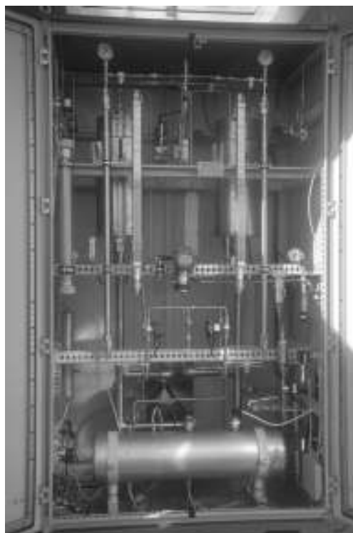
Figure 3-11 The PURE Energy Centre electrolyzer.
