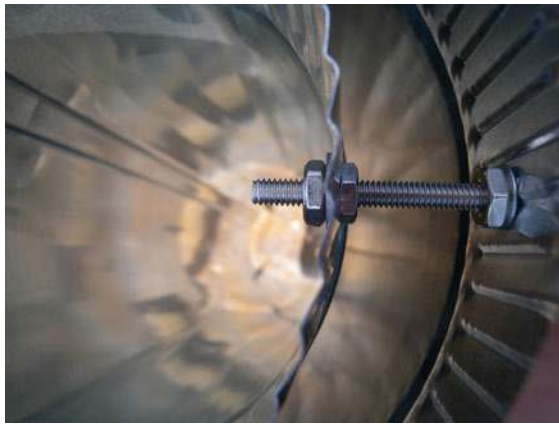
Figure 8-31. Suspending the 6 in pipe inside of the 8 in pipe produces a heat barrier and makes for safer operation.
