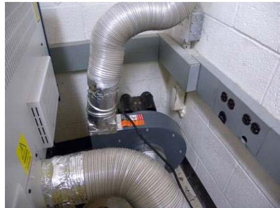
Figure 6-16. Ventilation systems require a substantial amount of space and generate a lot of noise. Ensure your Makerspace has allocated the necessary resources for this system.
