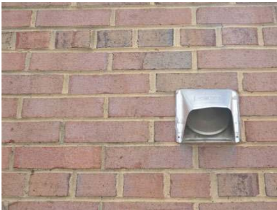
Figure 1-4. The ventilation system directs unwanted fumes outside of the building.
