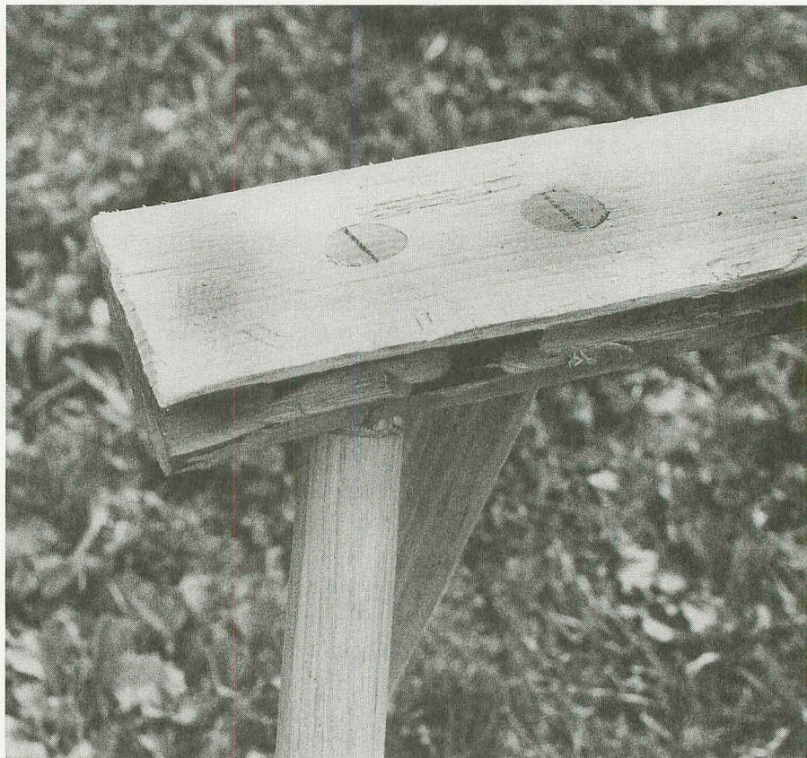
The tenon wedges must be perpendicular to the long fibers of the trestle.
