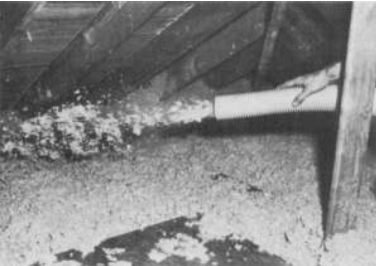
Figure 8-4 Fill insulation (mineral wool) being blown into attic. (Courtesy of Mineral Wool Mfg. Assn)
