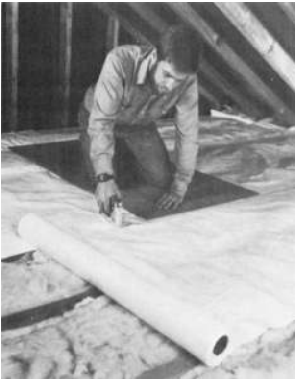
Figure 8-17 A product from Du Pont called Tyvek is being used to cut air infiltration in an attic. The product is stapled into place.
