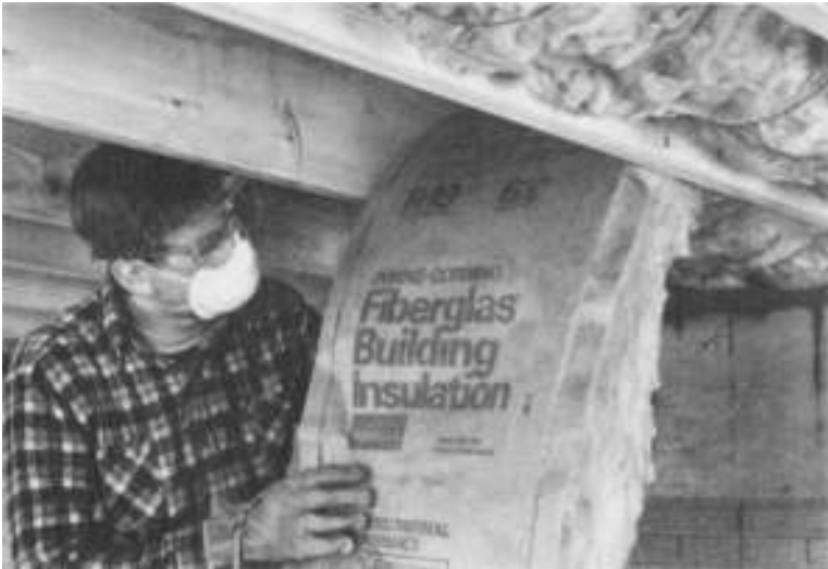
Figure 8-15 Fit blankets between floor joists and hold in place with flexible wire rods. (Courtesy of Owens-Corning)
