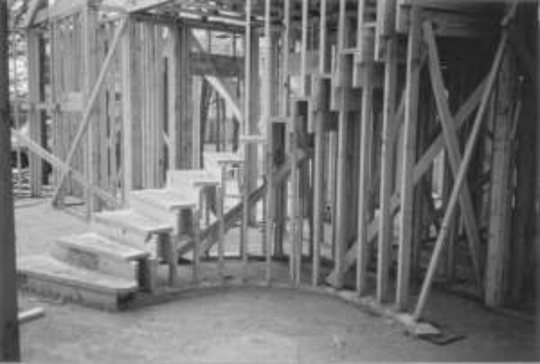
Figure 1-20 Note the curved portion of the stair case attached to the floor.
