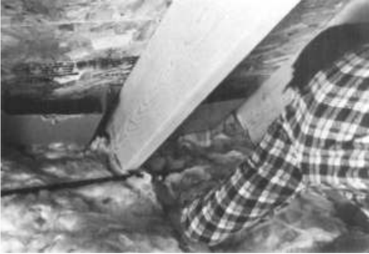
Figure 8-11 Installation in attic floor. Start with installation of proper vent to soffitt space under eaves. These vents are made on-site of corrugated cardboard and stapled onto roof sheathing. Next, tuck fiberglass blankets against vents between rafters and joists. (Courtesy of Owens-Corning)
