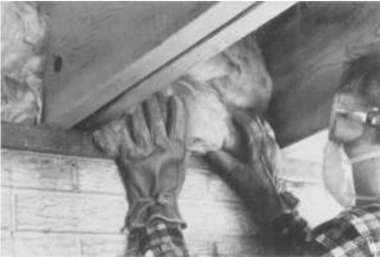
Figure 8-14 In the basement, tuck insulation above the sill between and along joists. (Courtesy of Owens-Corning)
