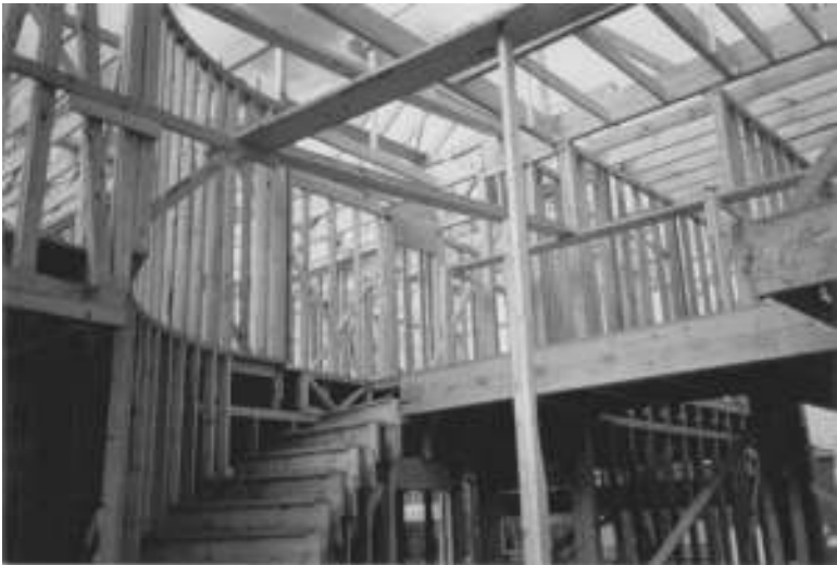
Figure I-19 Most of the house has been framed and the stairs are in place.
