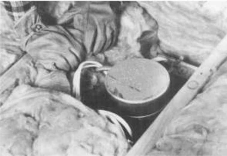
Figure 8-12 Light fixture. To prevent fire, keep insulation at least 3 inches away from recessed light fixtures unless the fixture is rated "I.C." for direct contact of insulation in an insulated ceiling. (Courtesy of Owens-Corning)
