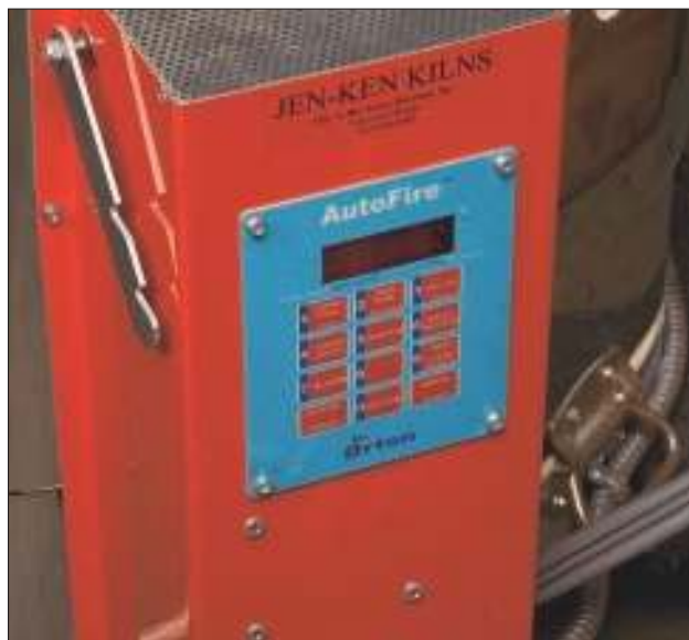
Figure 13-2: Automatic controller mounted on a glass kiln.
