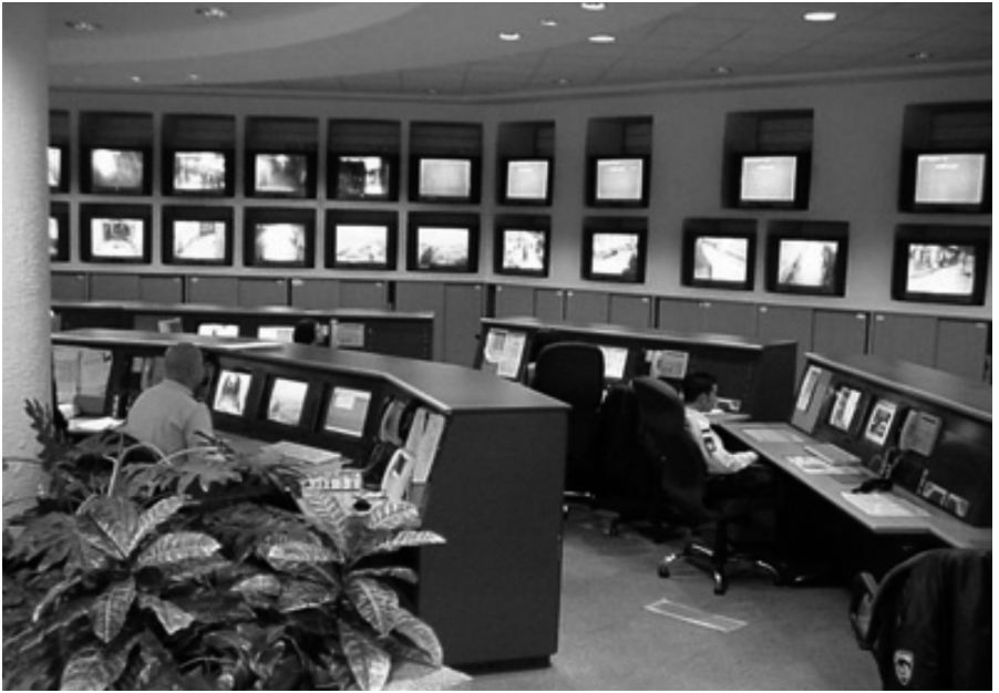
Figure 10.2 Mabat 2000 control room in the old city of Jerusalem
