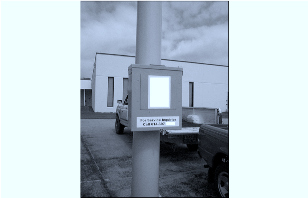
Figure 3.2 The Drop Box Installed
