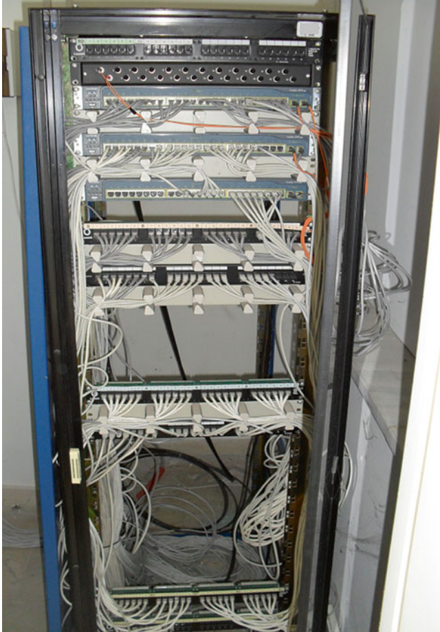
Fig. 3.7 Rack with patch panels
