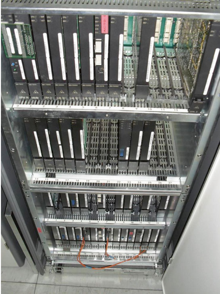
Fig. 1.2 The front side of the PBX
