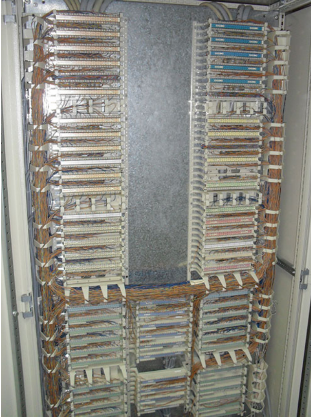
Fig. 3.6 Large company main distribution frame
