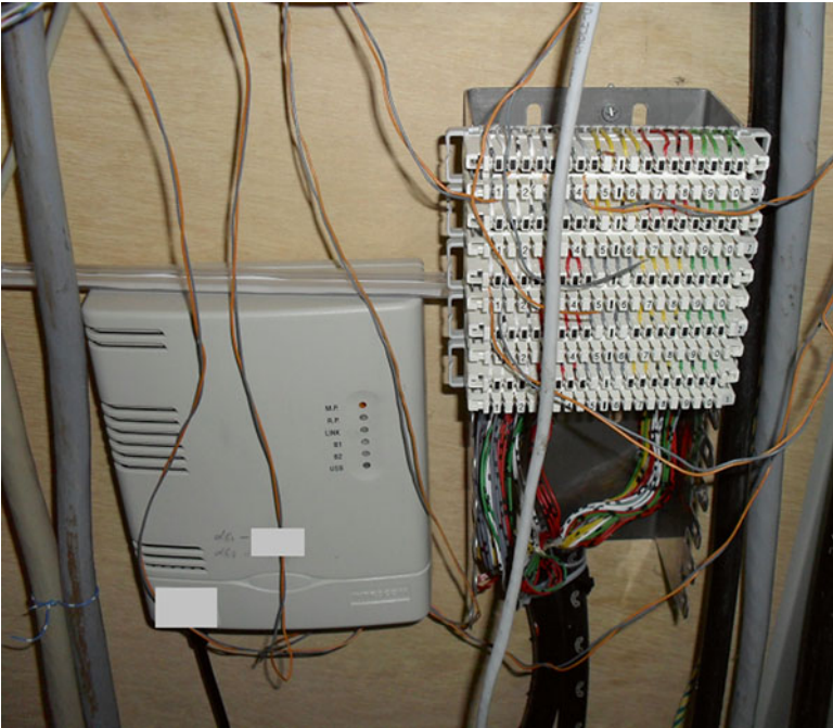
Fig. 3.4 Small office main distribution frame and CPE
