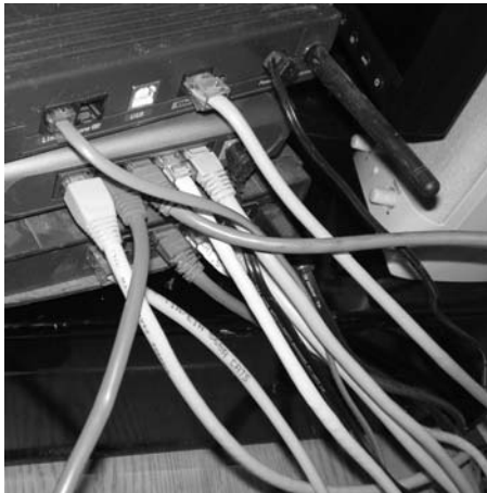
Figure 3-6: The cables connected to your network controls can often form a confusing mess.
