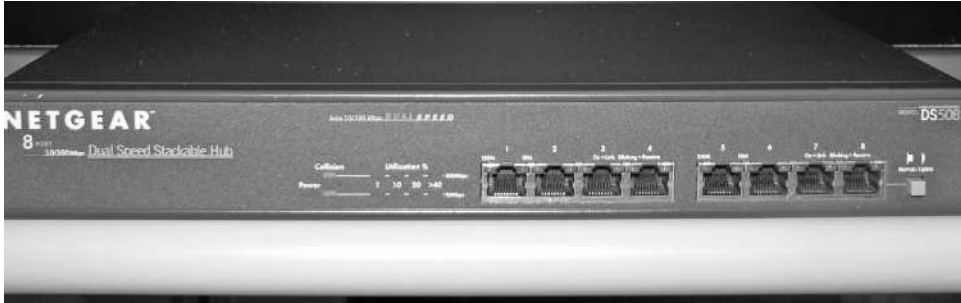
Figure 2-4 A typical hub with indicator lights
