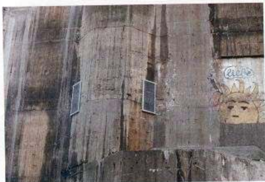
Concrete Worn: Cast Concrete
