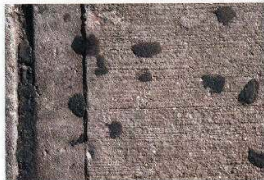
Concrete Worn: Poured Concrete Sidewalk
