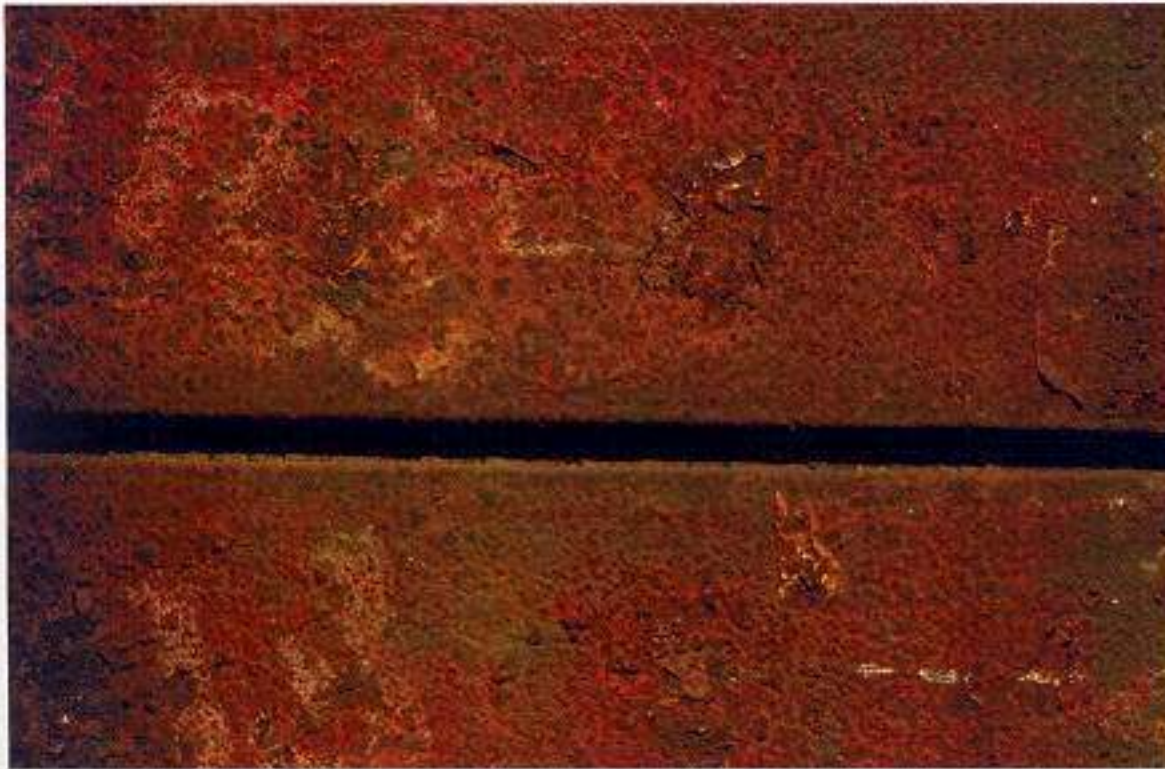
1.4 Rusted metal (Photo courtesy of Brian Drucker).
