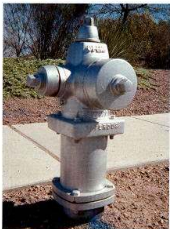
1.5 Fire hydrant in an Arizona suburb.
