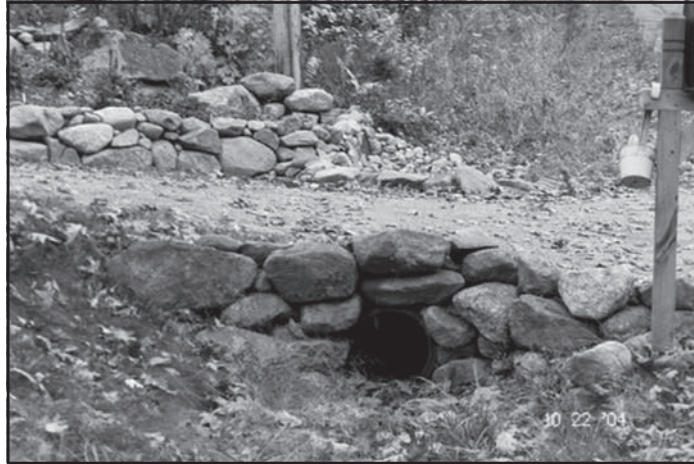
Figure 59—Culverts are a good option for moving small volumes of water under a trail.
