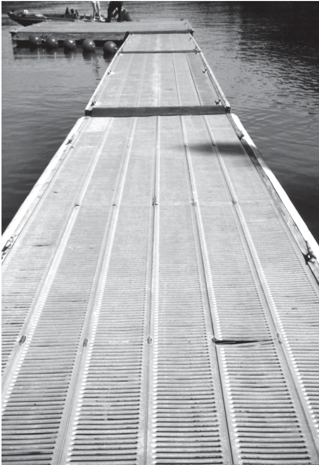
Figure 4—This dock at Dworshak Reservoir in Idaho uses metal grating as its deck. Metal decking provides drainage and traction but can still be slick when it is muddy and wet.
