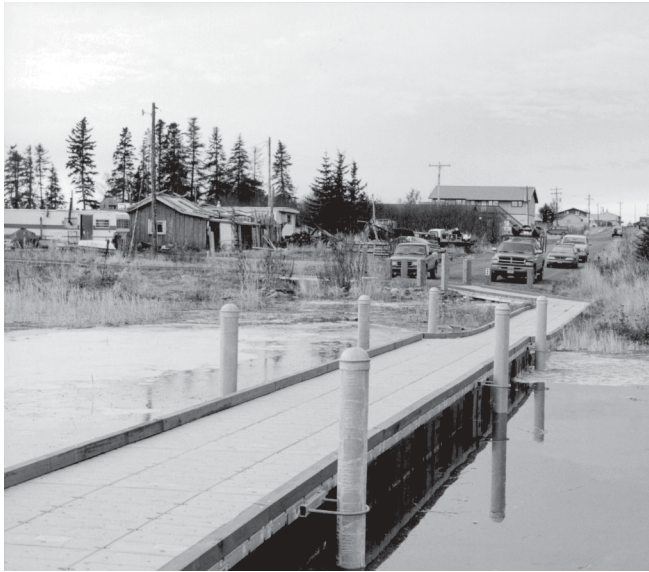
Figure 22—This dock uses multiple external pile holders for anchorage (photo by Paul Schrooten, USDI Fish and Wildlife Service).
