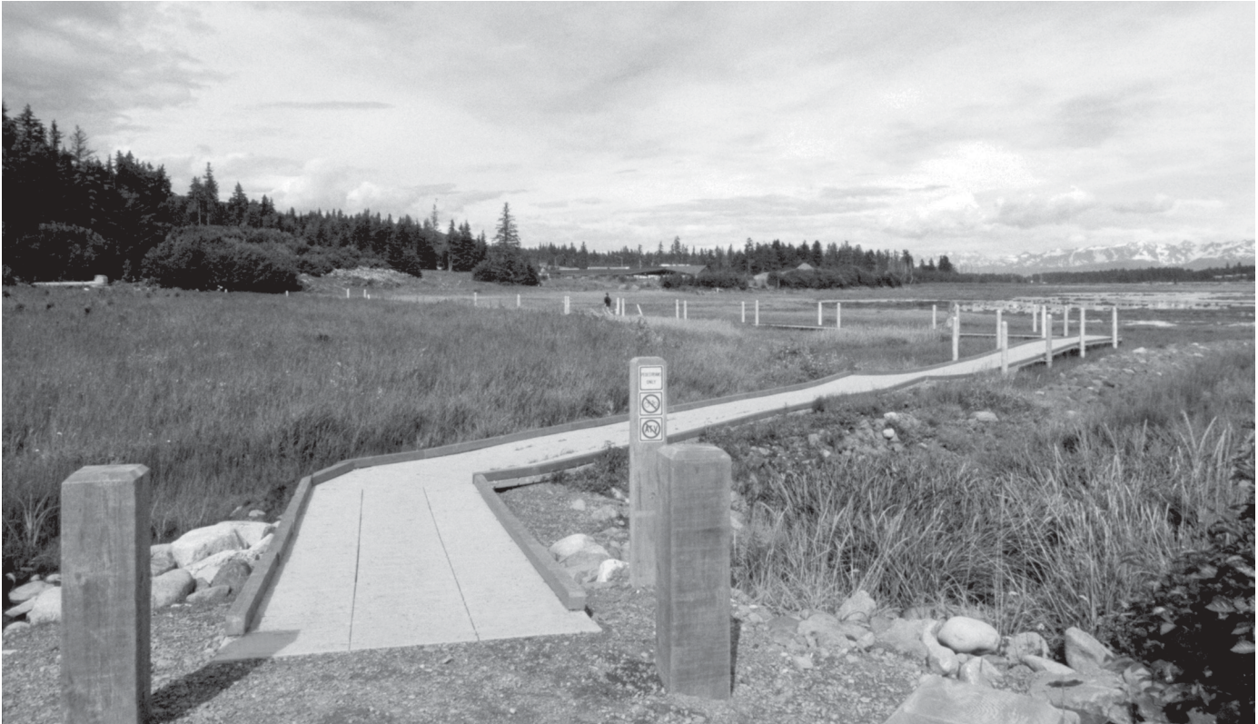
Figure 8—This floating bridge crossing a wetland in Alaska uses the Superdeck modular system (photo by Paul Schrooten, USDI Fish and Wildlife Service).
