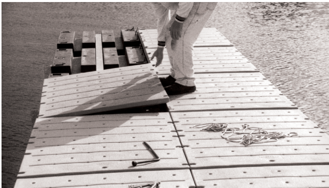
Figure 1—This commercially available modular dock system is easily assembled using common tools (photo by Paul Schrooten, USDI Fish and Wildlife Service).
