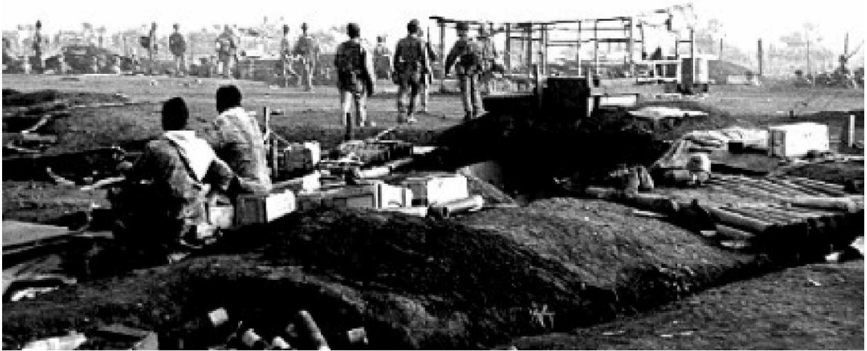
Members of Special Forces Detachment A-14 supervise construction of defenses in the hamlet of Chau-Lang during December of 1962 (US Army)
