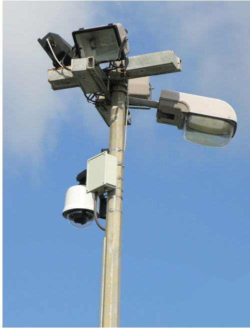
Figure 15.17 An example of a pole-mounted enclosure.
