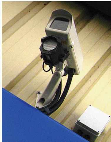
Figure 3.20 An IR-sensitive network camera with an IR illuminator attached below the camera housing.
