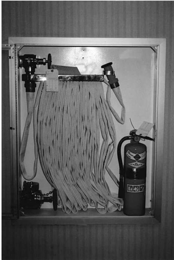
Figure 8-3 ■ Wall cabinet containing standpipe system, hose, and fire extinguisher.
