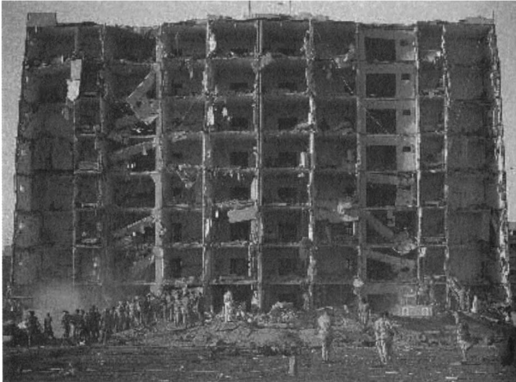
Figure 18-5. A photo of bombed Khobar Towers building. A terrorist attack on a peacekeeping force in Dhahran, Saudi Arabia, left 19 dead and hundreds injured.
