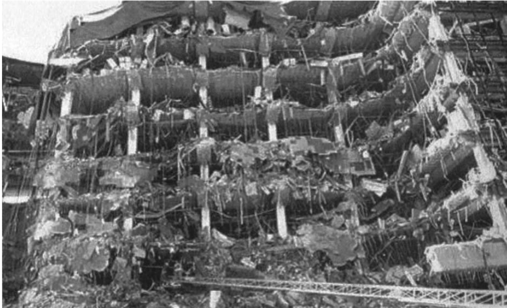
Figure 18-1. Photo of bomb destruction at Oklahoma City Federal Building. The bombing of a federal building in Oklahoma City delivered a tragic reminder to Americans of the cruelty of terrorists.
